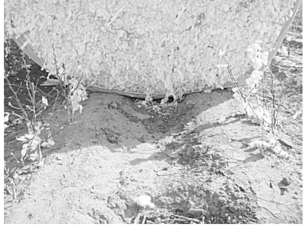
Incorrect Staging Surface
